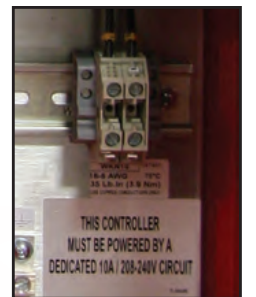
• Incoming power connection
