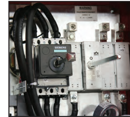
• Isolating switch and circuit breaker
